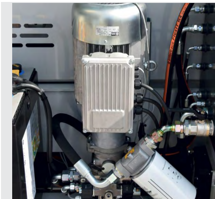
A/C electric power unit
