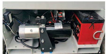
AGM batteries to ease maintenance. New disposition of hydraulic components on the lower frame which integrates forklift pockets.
