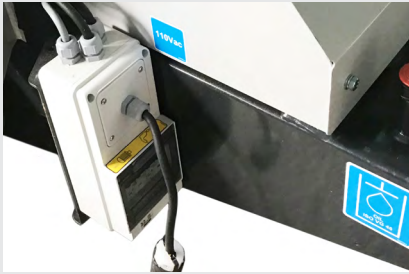
Thermal-magnetic switch panel and power line inlet.
